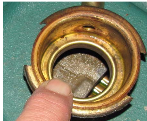
No coolant visible in heat exchanger
