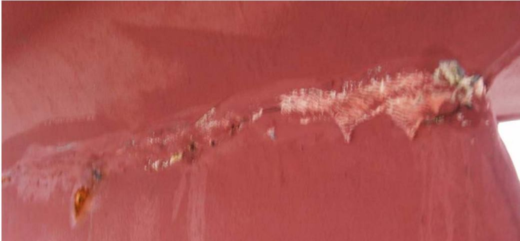
Crudely caulked and weeping keel / hull joint.
