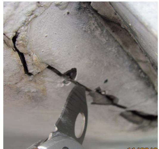
Fracture under port swim platform hydraulic arm
