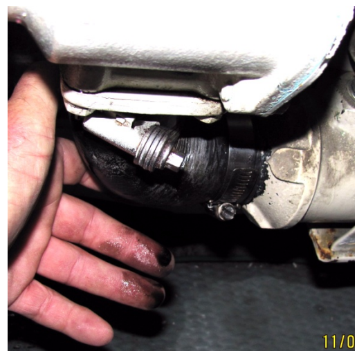
Oil leak at oil cooler close to raw water pump on port engine.
